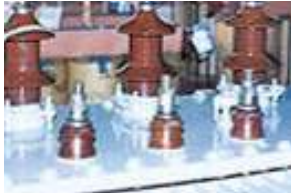
HV bushing with terminal connectors
